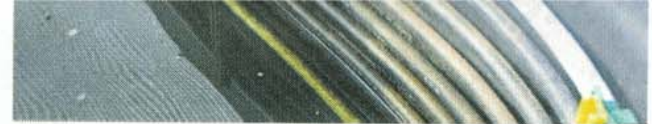
Heating elements inside a fish tank, more effective than simply using the air in the greenhouse.
